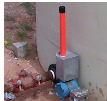
SFRSS HART Node Connected to a pressure sensor for tank level monitoring
