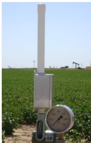
SFRSS A2 Powering and Monitoring a 4-20 mA Pressure Sensor on an injection well
