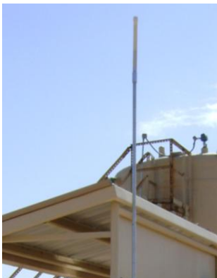
SignalFire Gateway-in-a-Stick connected to an RTU at a tank battery
