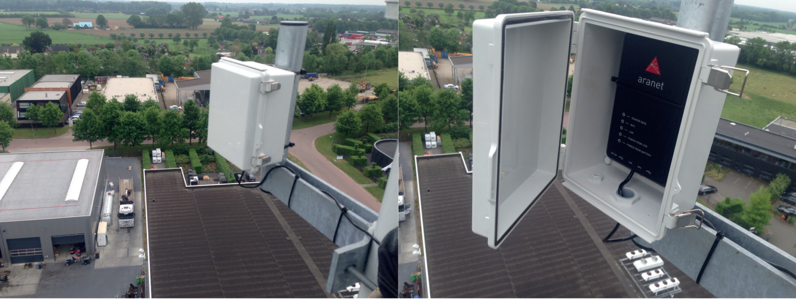
Aranet PRO 100 gateway in a weatherproof container at 38m/124.7ft.
